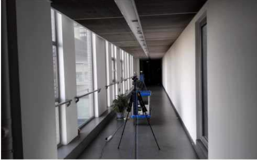
FIGURE 7. The photo for the measurement environment of the corridor.
