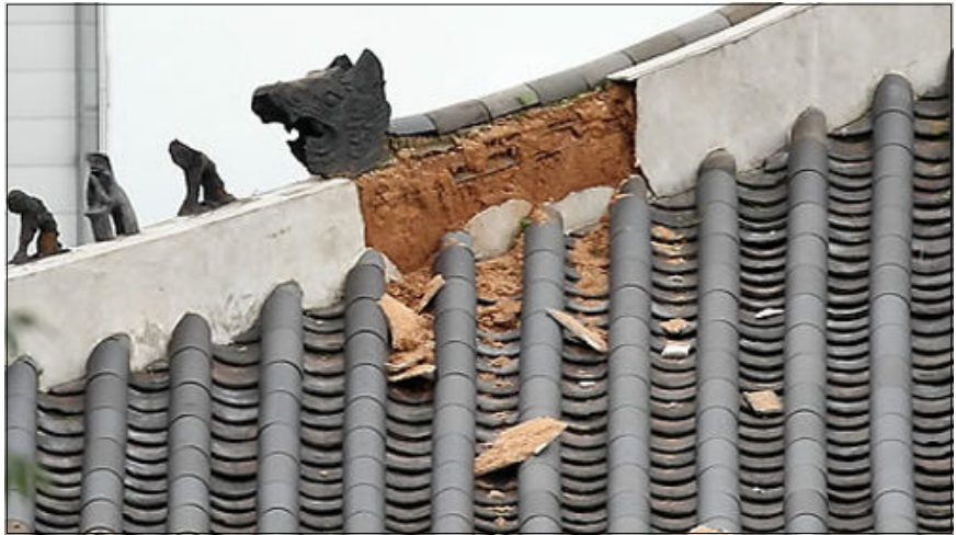
Fig. 2. Heunginjimun roof damaged by heavy rain (Kwon, 2011)
